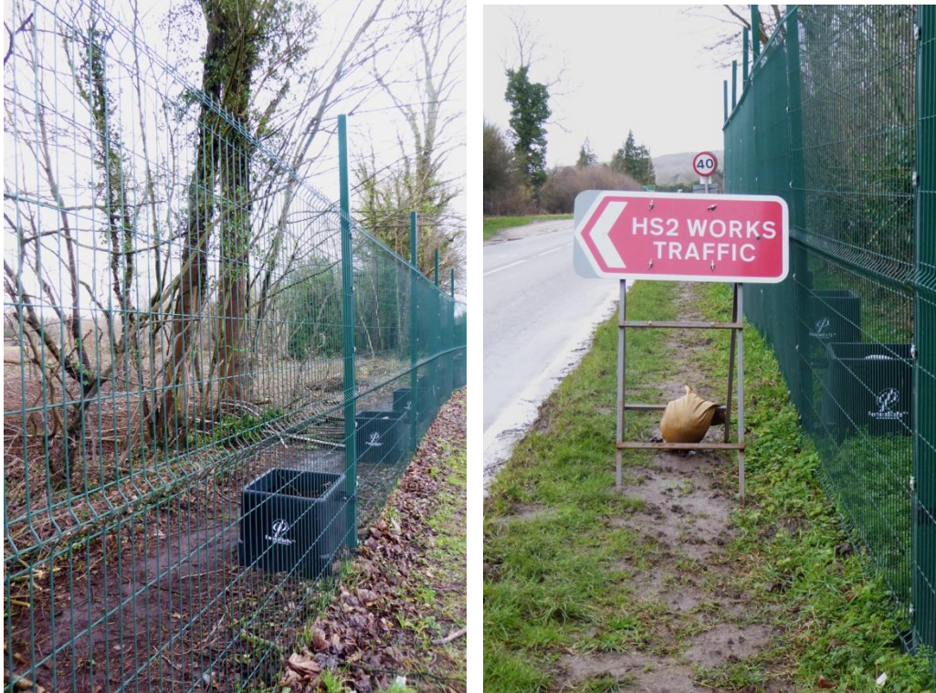
West side – the security fencing, constructed on the existing footpath; further gratuitous obstruction of the limited space remaining, by a roadsign
