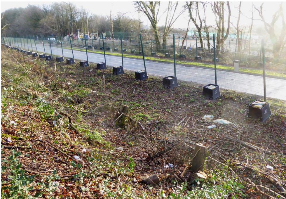
The security fence is 2 to 3 metres inside the railings marking the edge of the highway.
