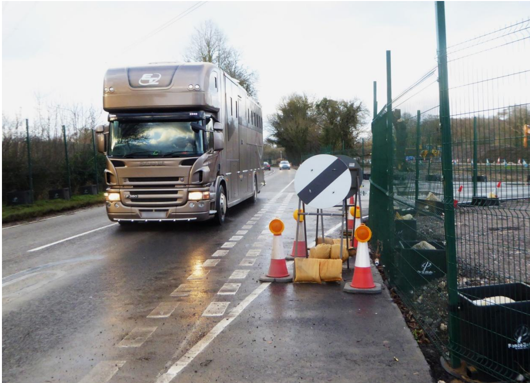
Such as this carelessly positioned road sign
